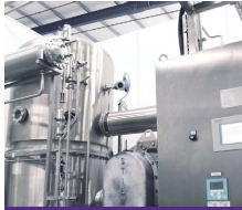
On-site blending tanks
