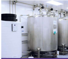
On-site WFI production
